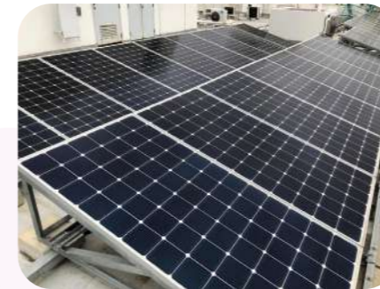
天台太陽能板 Solar Panels on the roof
